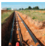
Pipelines in France. © Ineke Scholte
